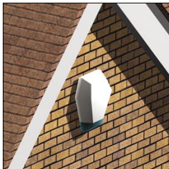
Front active alarm bell box
